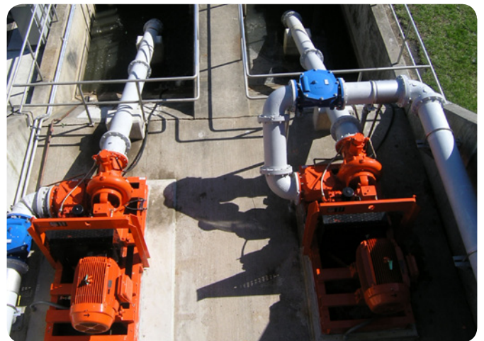
Two permanently installed 12" DPC300 electric drive pumps moving effluent from a secondary trickling filter to a chlorination chamber, then to discharge.
