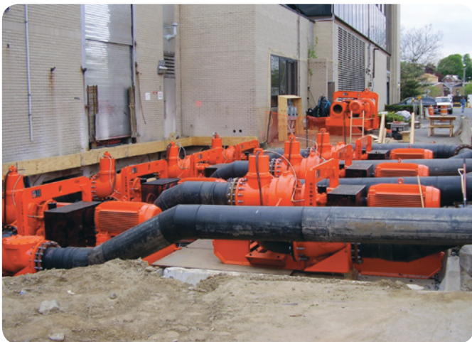
Eight 18" CD400M electric drive pumps (some benched four feet down) are positioned to pump product out of an influent chamber.
